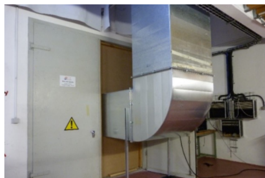
Photo 2 : Aspiration section outside the reverberant room (2, 3 & 4)
